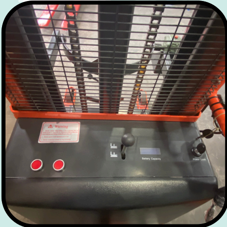
ELECTRICAL LIFTING CONTROL PANEL
